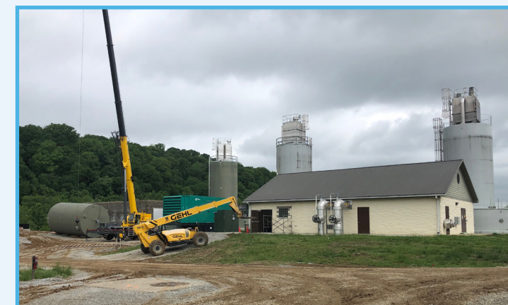
Construction underway for a new water treatment plant at River Ridge Commerce Center in Jeffersonville, IN
