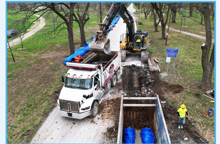
Louisville Water installed two residual lines on River Road well ahead of schedule
